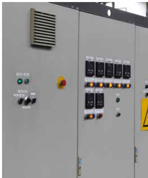
Switch cabinets for line control
